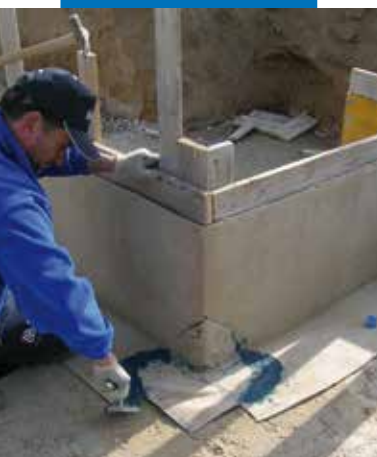
Grouting a gap in correspondence with a corner of the sheet with Mapeproof Mastic
